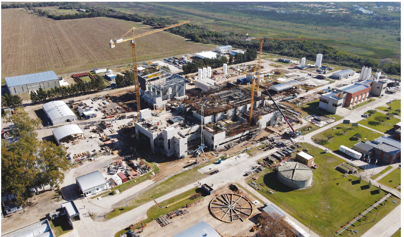
Construction has paused on the small modular reactor CAREM, shown here in 2023 at the outskirts of Buenos Aires.
