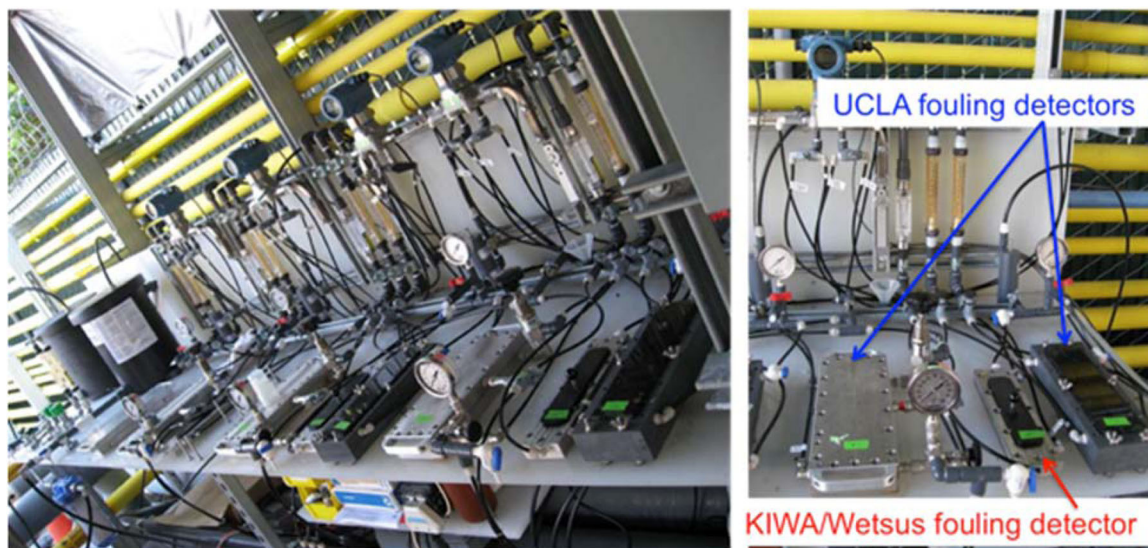
Fig. 11 Pictures of various fouling detectors employed at a seawater desalination plant. Research conducted at the Long Beach Water Department's seawater RO/NF demonstration plant focusing on NF/RO membrane biofouling mechanisms, prevention, and monitoring. Tanuwidjaja 107 compared three different membrane fouling detectors to understand potential bias due to different monitoring device configurations. At left, four parallel trains of 3 sensors per train are depicted. At right, a single train of 3 fouling detectors including UCLA's high-pressure fouling detector, which enables flux, rejection and differential pressure to be monitored as well as a UCLA low-pressure fouling detector and a KIWA/Wetsus low-pressure fouling detector; both low-pressure fouling detectors monitor differential pressure only. Original image courtesy of Dian Tanuwidjaja. Copyright University of California, Los Angeles.
